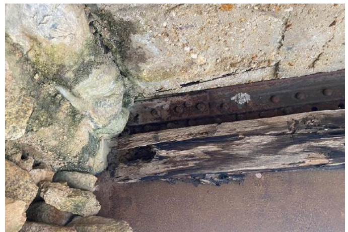
Above: Underside of bridge, showing bridge defects of rust pitting of the girder, water ingress into the bridge structure and exposed and rusted reinforcement bars in the decking.
