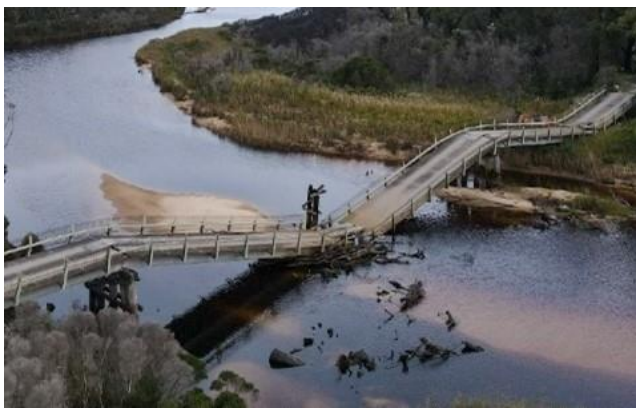
Fire damaged Thurra River Bridge
