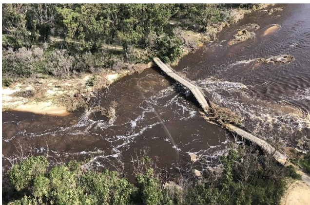
Flood damaged Thurra River Bridge
