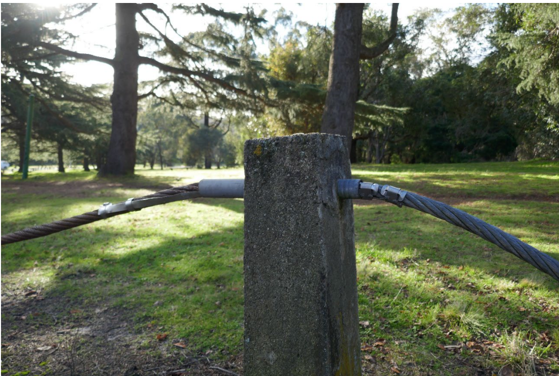
Figure 59 Evidence of previous efforts to make-good failed sections of cabling
