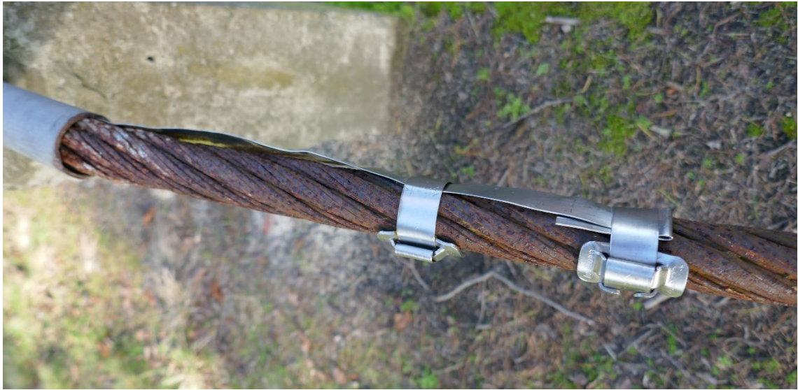
Figure 60 Evidence of previous efforts to make-good failed sections of cabling
