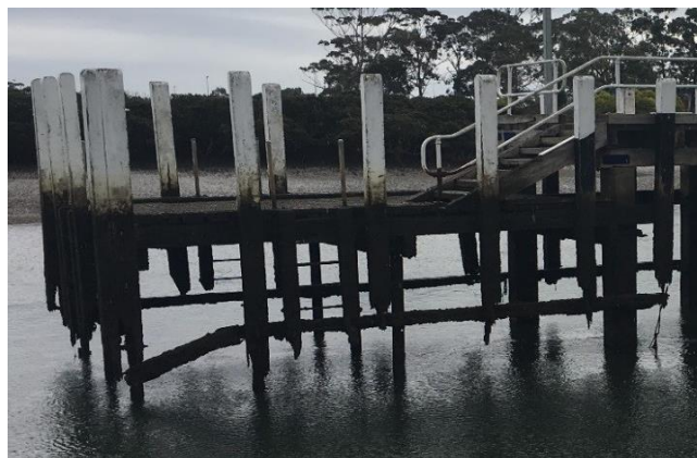
Current poor condition of fenders and walers.
